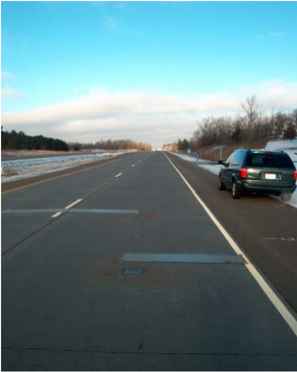
Figure 13-1 Pavement Condition in the Downstream Direction at 550100
