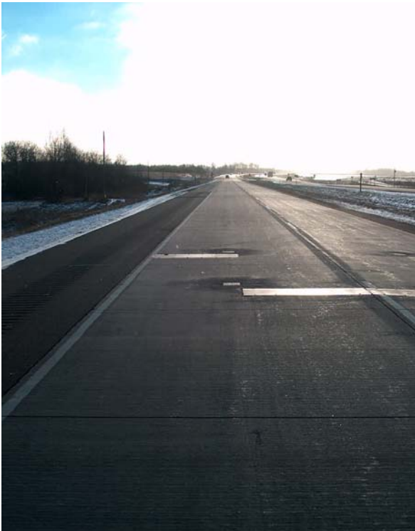
Figure 13-2 Pavement Condition in the Upstream Direction at 550100
