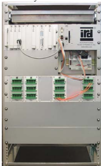
Figure 3 - Typical electronics system hardware
