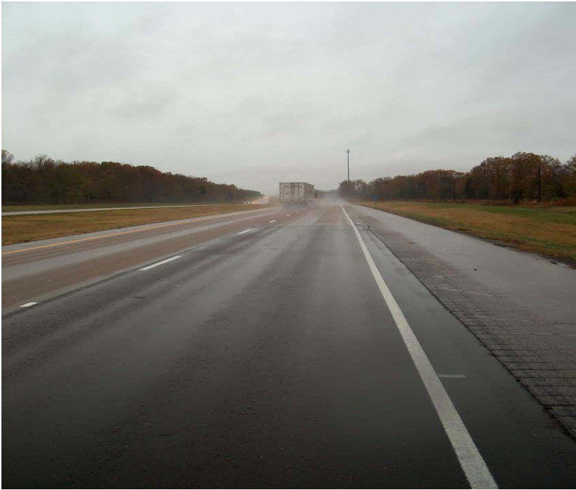
Figure 13-1 Pavement Condition at Site 470600 (Downstream)
