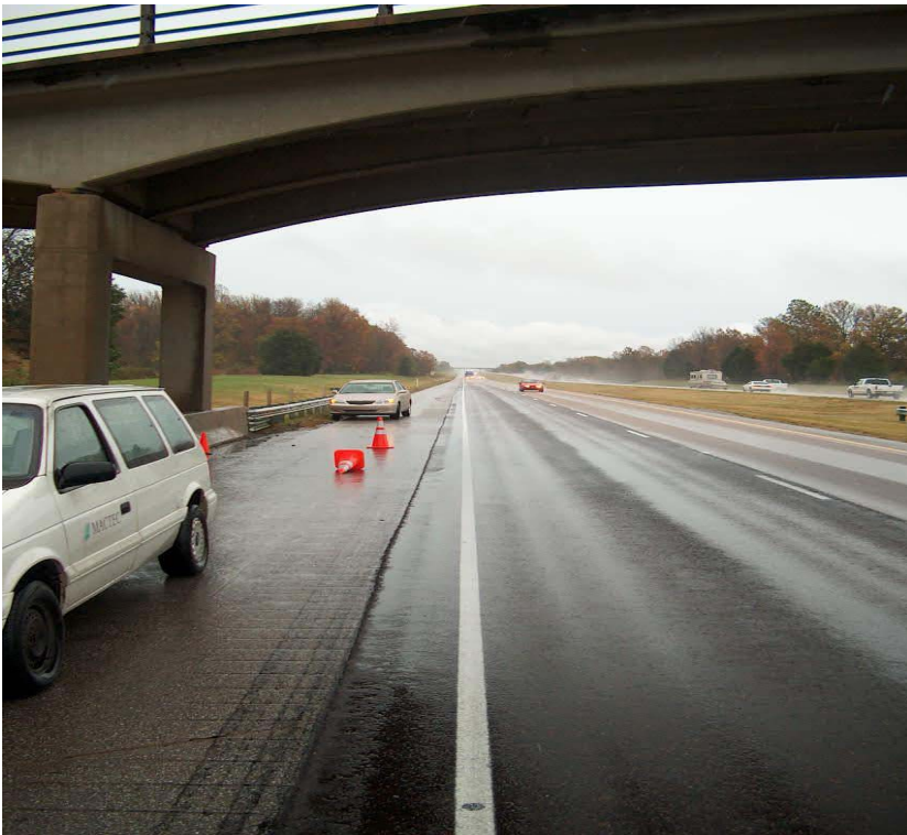
Upstream_1_TO_1_47_5A_0600_11_18_03.JPG (Distress Photo 2)
