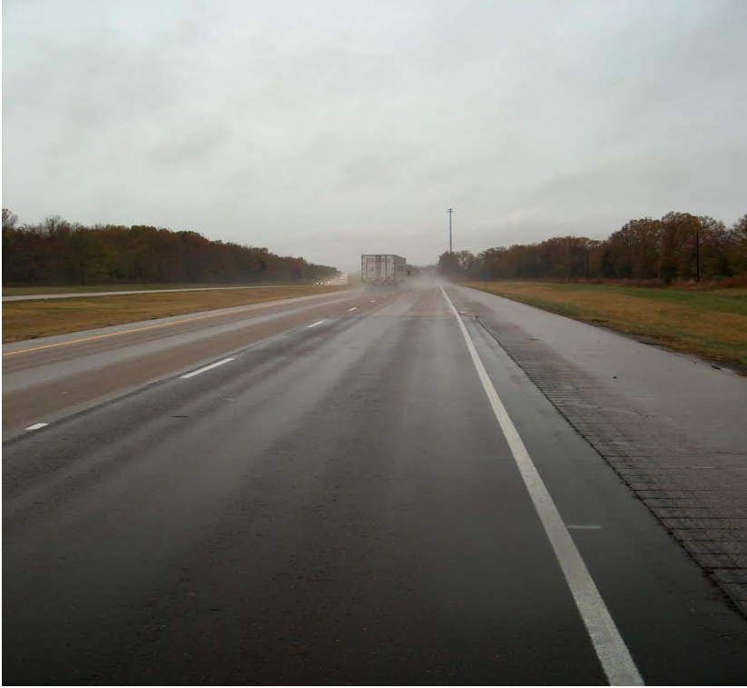
Downstream_1_TO_1_47_5A_0600_11_18_03.JPG (Distress Photo 1)
