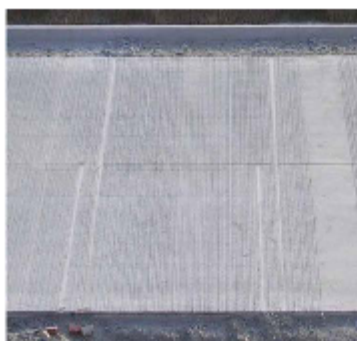
1. Lineas sensors installed in concrete
