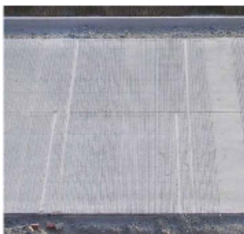
1. Lineas sensors installed in concrete
