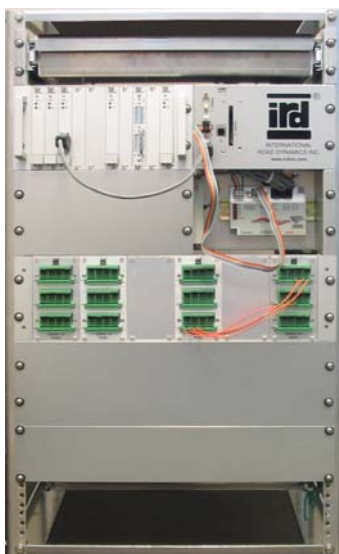
Figure 3 - Typical electronics system hardware
