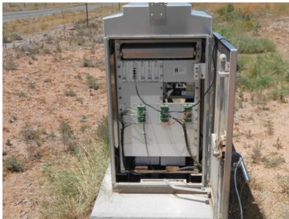
Photo 2 – Cabinet Interior (Front)
