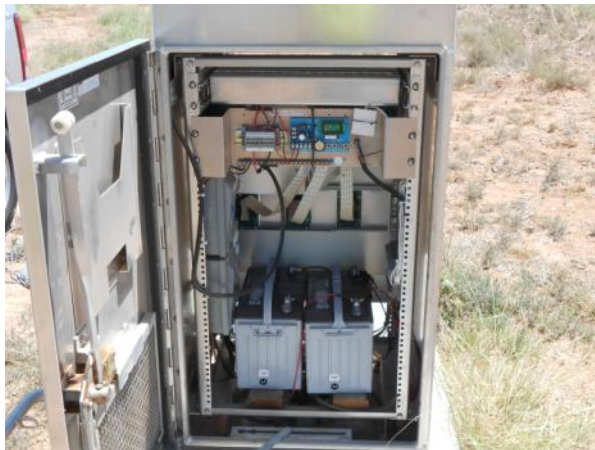
Photo 3 – Cabinet Interior (Back)
