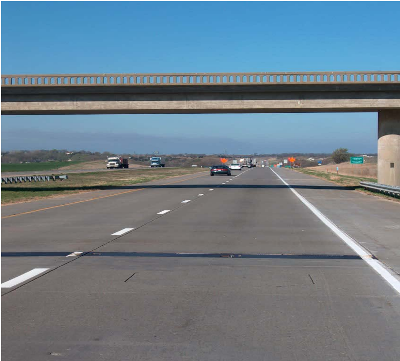
Downstream_TO_4_20_30A_0200_3_31_04.JPG (Distress photo 1)
