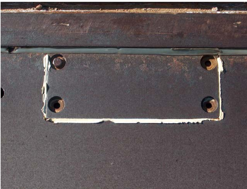
Figure 15-4 Missing Bolts in Weight Sensors at 200200
