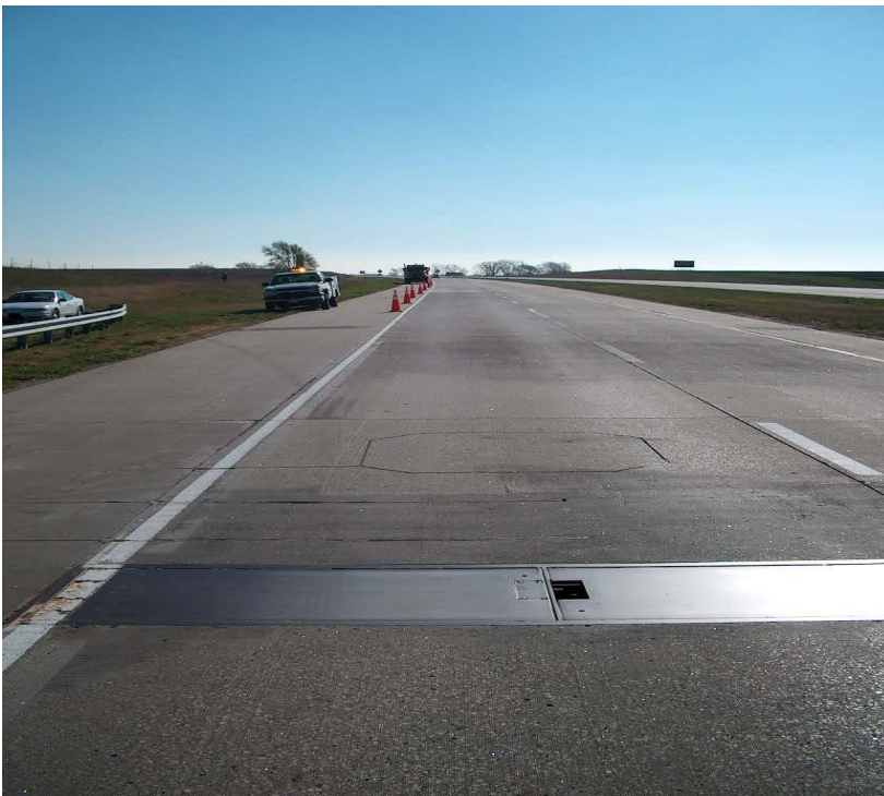
Upstream_TO_4_20_30A_0200_3_31_04.JPG (Distress Photo 2)
