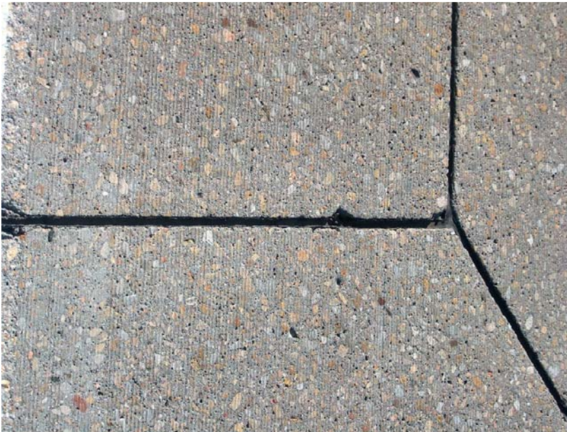
Figure 15-1 Insufficient Loop Sealant at 200200
