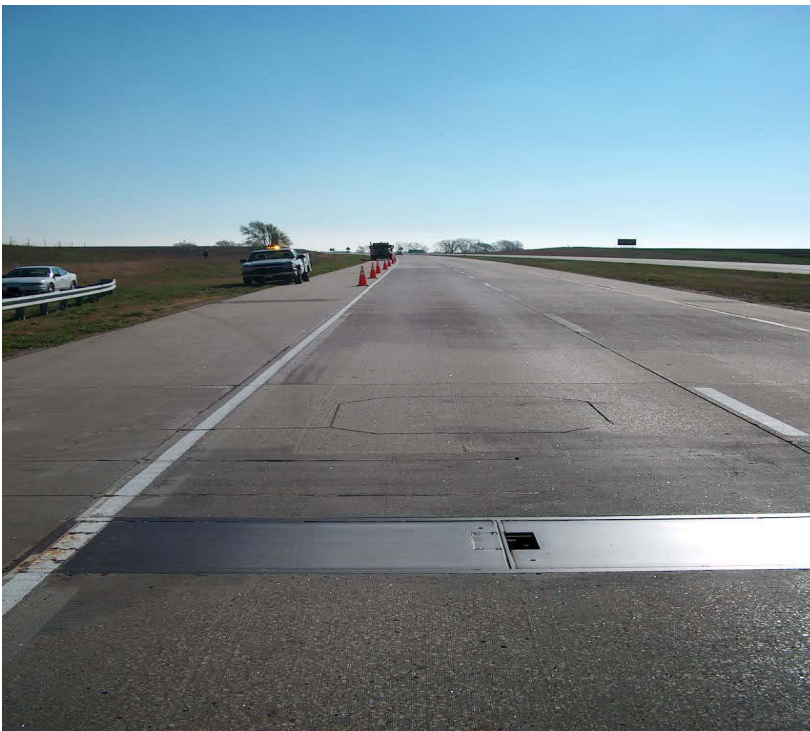
Figure 13-2 Pavement Condition in Upstream Direction at 200200
