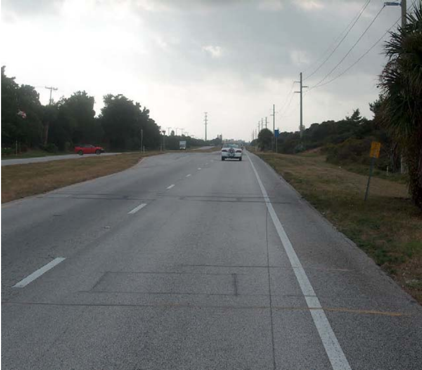
Downstream_TO_2_12_13A_0500_12_04_03.JPG (Distress Photo 1)
