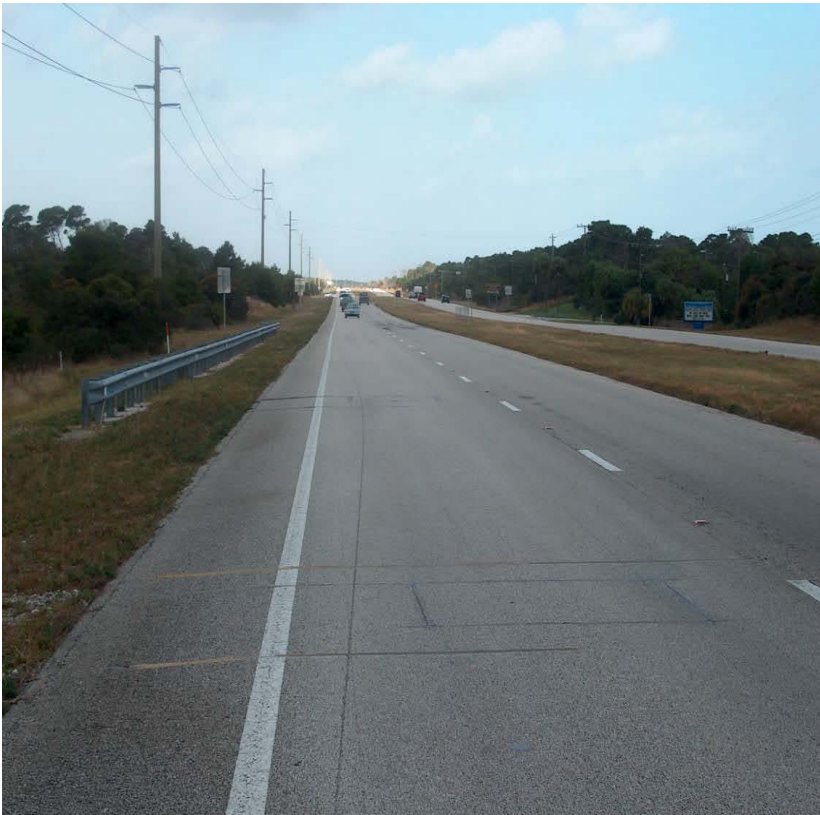
Figure 13-2 Pavement Condition of 120500 in Upstream Direction
