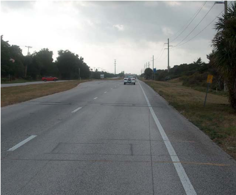
Figure 13-1 Pavement Condition of 120500 in Downstream Direction
