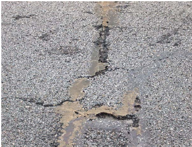
Figure 4-1 - Pavement Distress in Left Wheelpath – 120100 – 01 Mar 2005
