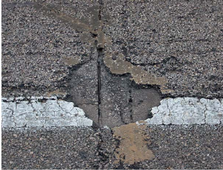
Figure 4-2 - Pavement Distress at Right Edge of Lane – 120100 – 01 Mar 2005
