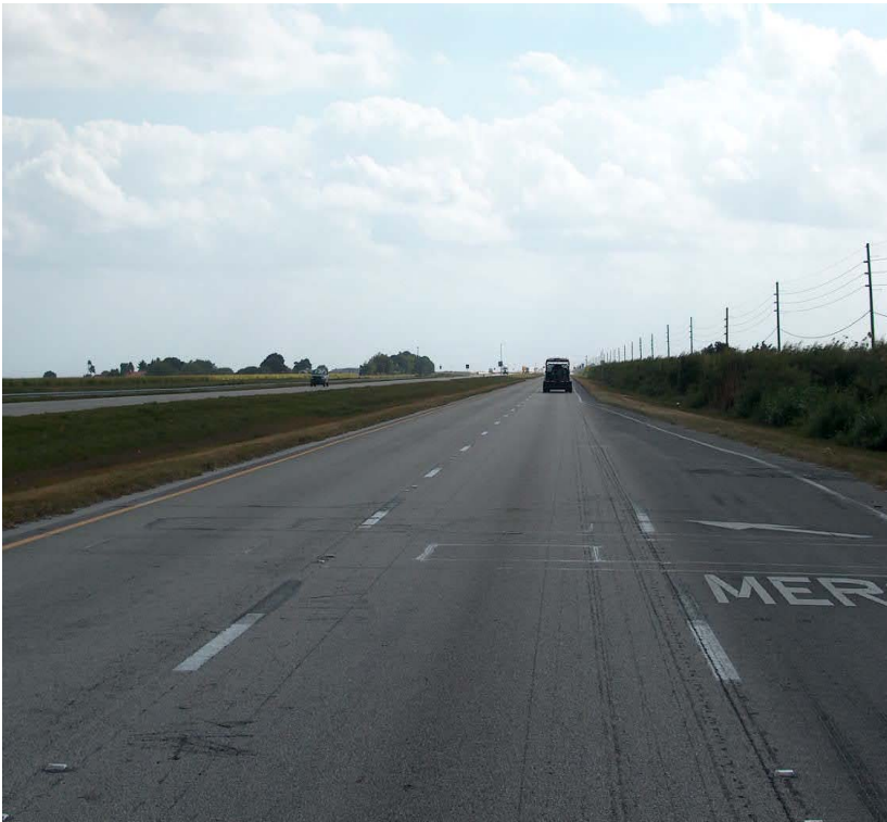
Downstream_TO_2_12_12A_0100_12_03_03.JPG (Distress Photo 1)
