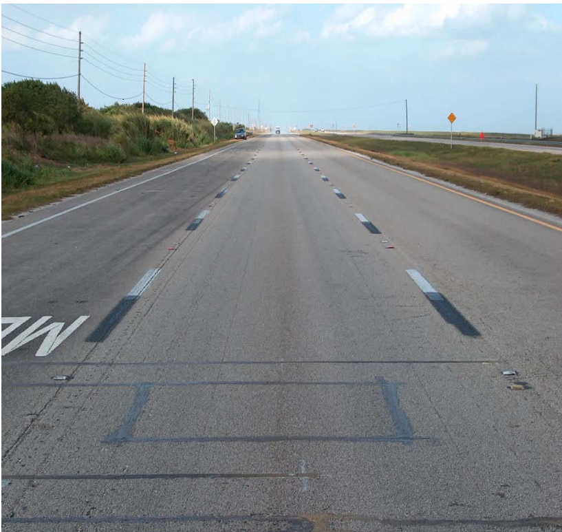
Upstream_TO_2_12_12A_0100_12_03_03.JPG (Distress Photo 2)
