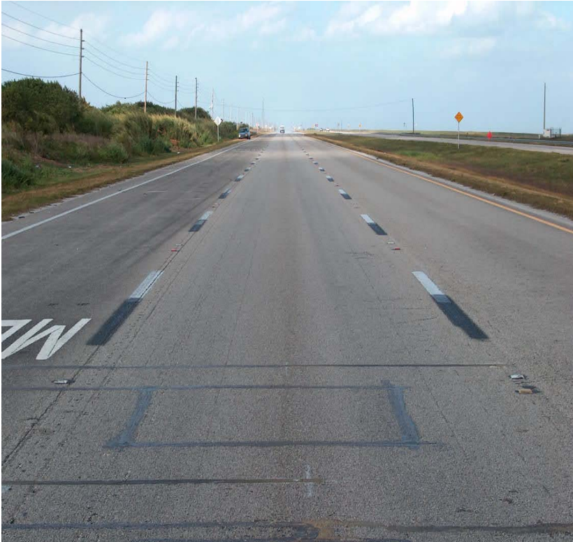
Upstream_TO_2_12_12A_0100_12_03_03.JPG (Distress Photo 2)
