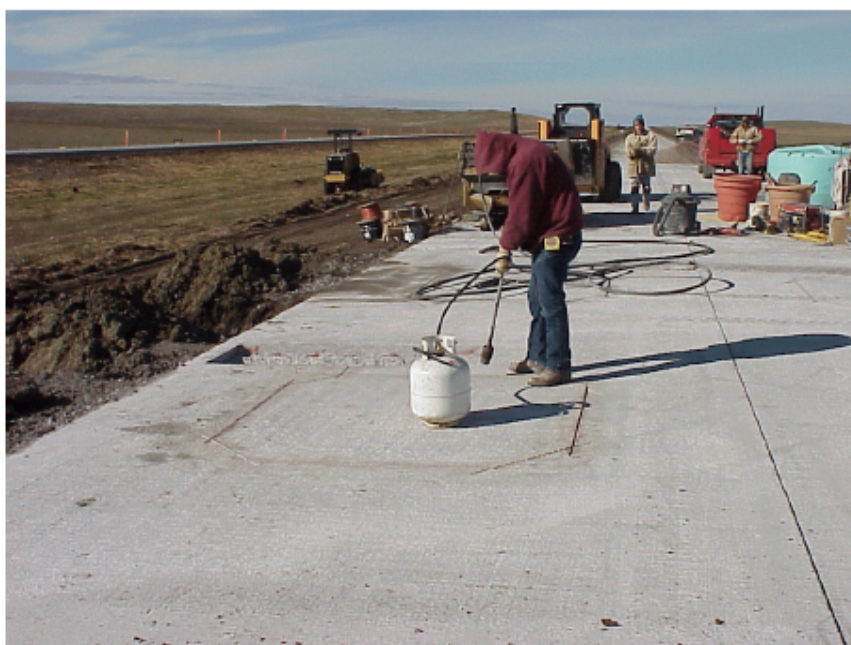
Figure 11 - Drying Recess with Propane 123-429-901-110.jpg
