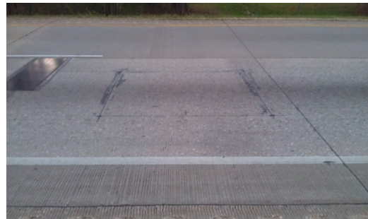
Photo 7 – Trailing Loop Sensor
