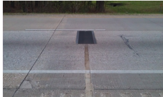
Photo 6 – Trailing WIM Sensor
