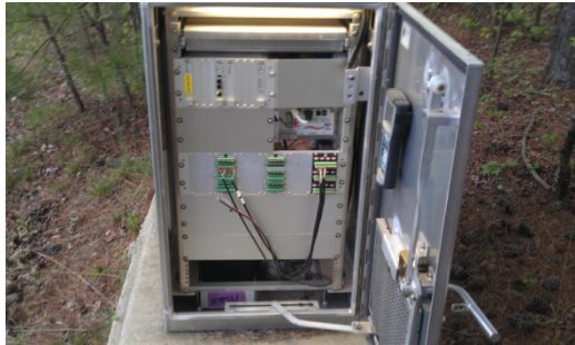
Photo 2 – Cabinet Interior (Front)
