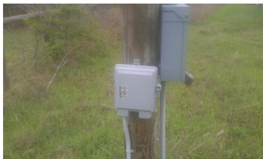
Photo 9 – Telephone Service Box
