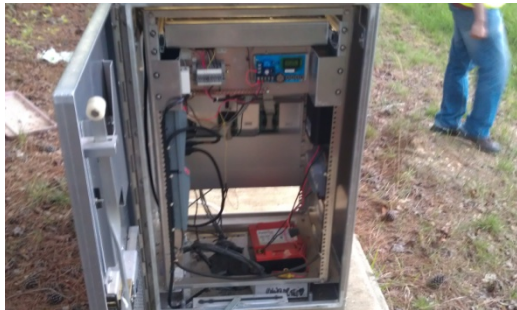
Photo 3 – Cabinet Interior (Back)
