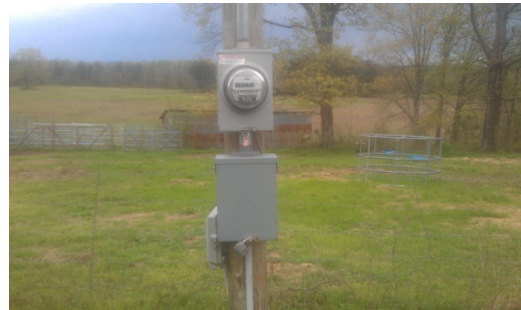
Photo 8 – Power Service Box
