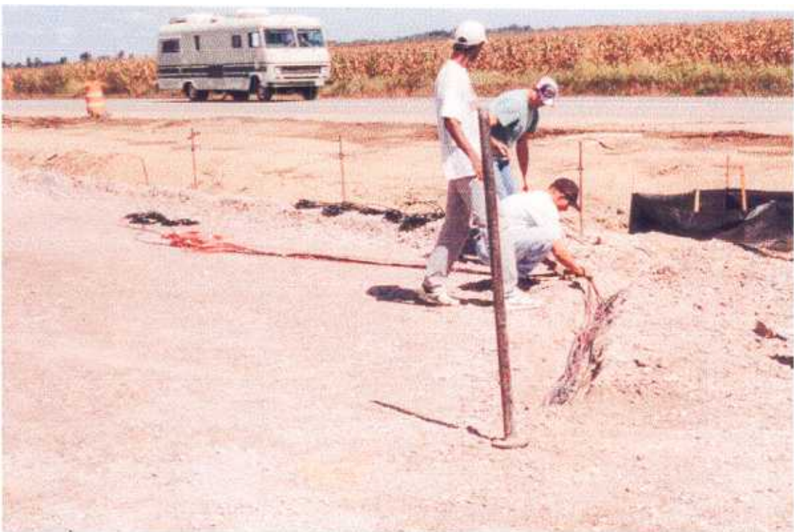
Photo 2 Wires from Probes at Instrumentation Hole
