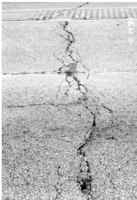
Figure 3. Pavement candidate for crack repair.
