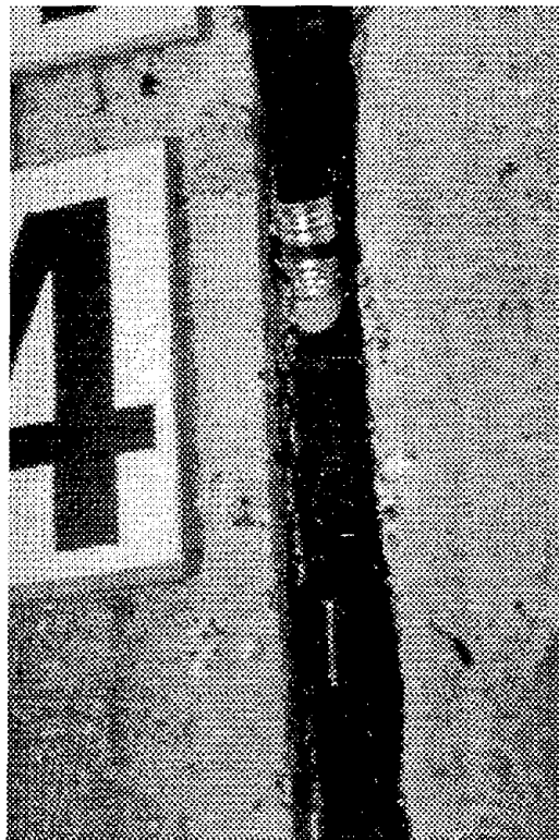
Figure 24. Partial-depth adhesion loss.
