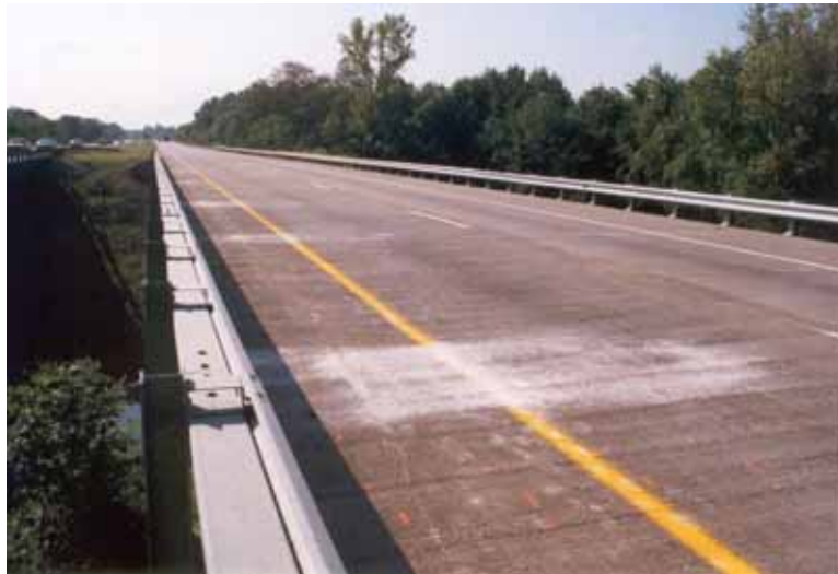
Figure 9. Photograph showing the eastbound deck of U.S. 52 over Raymond Run in Columbus, OH. The overlay is latex-modified.
