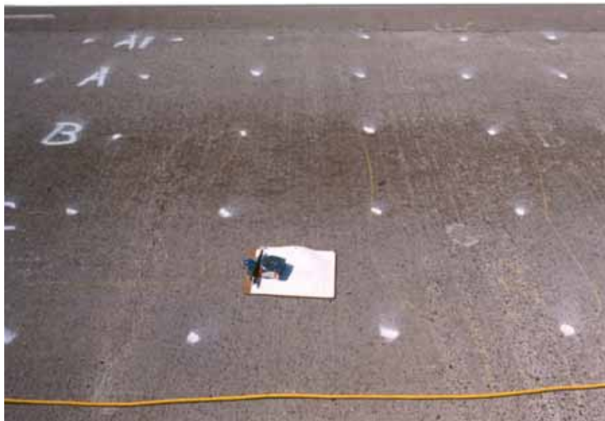
Figure 25. Photograph showing typical cracking found in the northbound deck of the U.S. 41 test section LMC.
