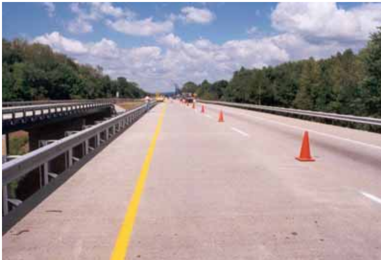
Figure 11. Photograph showing westbound passing lane of U.S. 52 over Raymond Run in Columbus, OH. The overlay is silica fume concrete.
