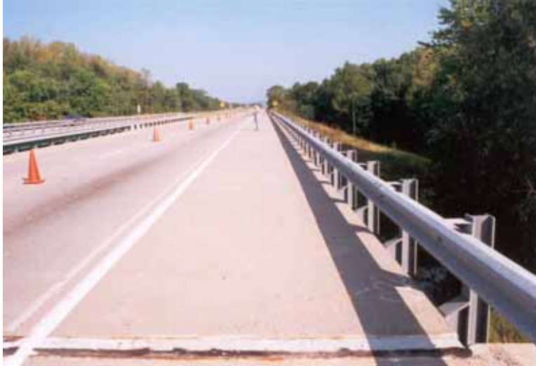
Figure 10. Photograph of westbound travel lane of U.S. 52 over Raymond Run in Columbus, OH. The overlay is latex-modified.
