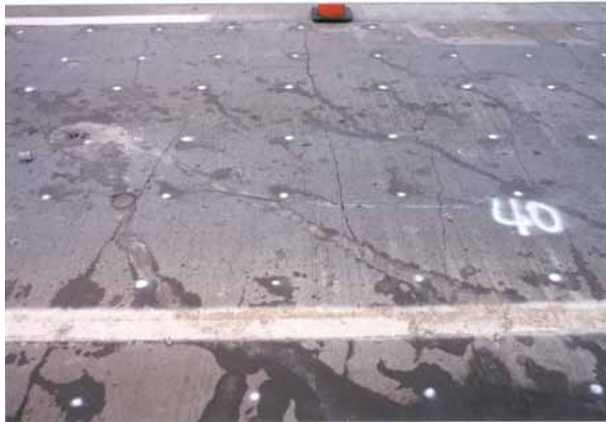
Figure 26. Photograph showing typical cracking associated with the southbound test section of U.S. 41 SFC.
