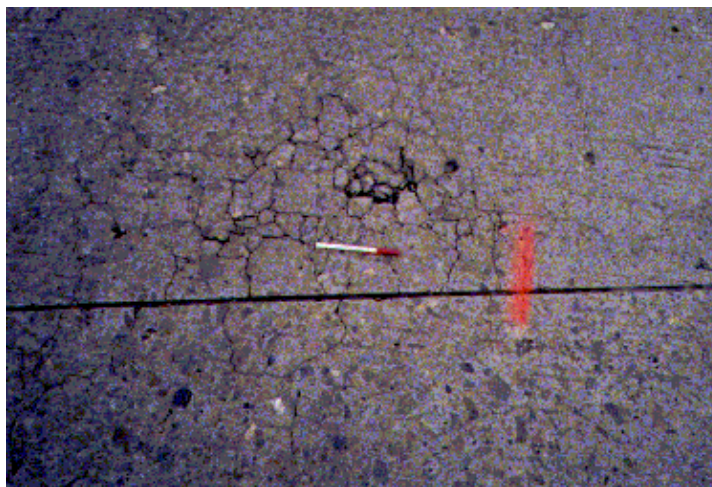
Figure 3. Joint distress of high severity (Winnemucca, NV).
