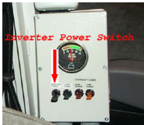
Figure 2.2.5.6. Remote switch for inverter power.
