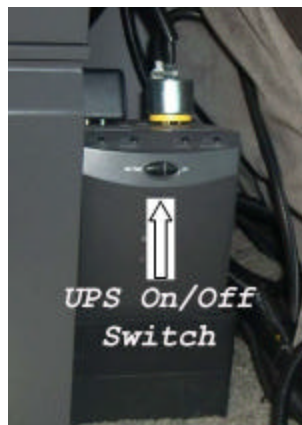
Figure 2.2.5.4. UPS on/off switch.
