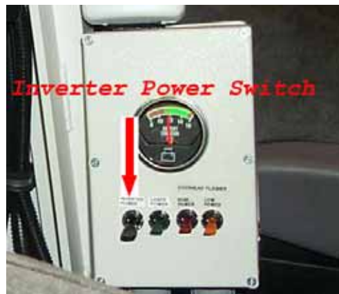
Figure 12. Photo. Remote switch for inverter power.
