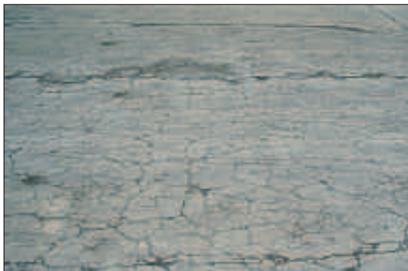
Figure 69: Distress Type JCP 8a – Map Cracking
