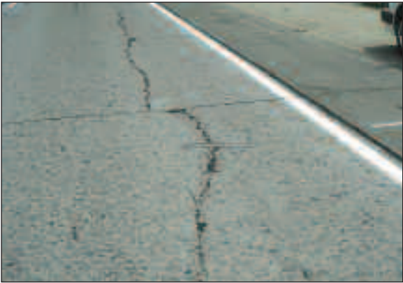
Figure 57: Distress Type JCP 3 High Severity Longitudinal Cracking
