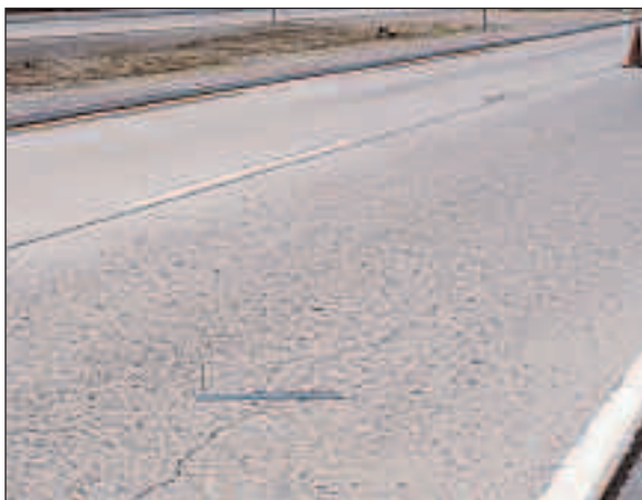
Figure 55: Distress Type JCP 3 Low Severity Longitudinal Cracking
