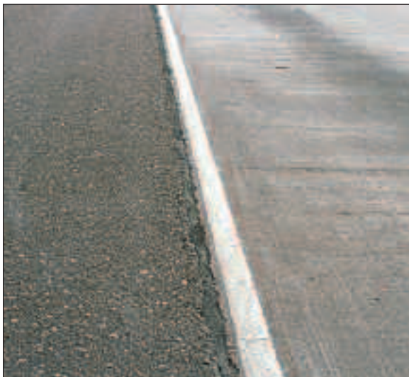
Figure 83: Distress Type JCP 14 Well Sealed Lane-To-Lane Separation
