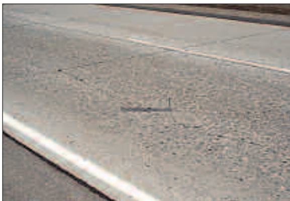
Figure 56: Distress Type JCP 3 Moderate Severity Longitudinal Cracking
