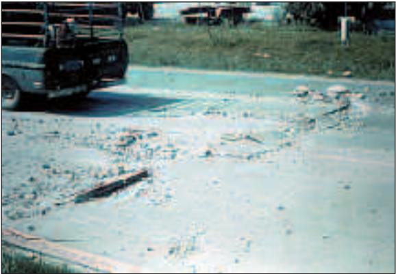
Figure 76: Distress Type JCP 11 – A Blowup
