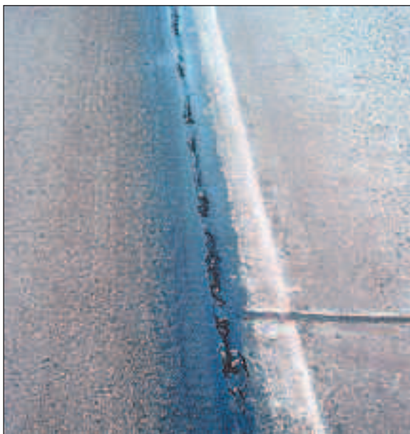
Figure 82: Distress Type JCP 14 Poorly Sealed Lane-To-Lane Separation
