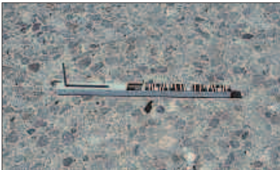
Figure 74: Distress Type JCP 10 - A Popout
