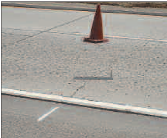
Figure 59: Distress Type JCP 4 Moderate Severity Transverse Cracking
