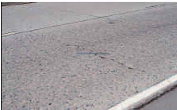
Figure 60: Distress Type JCP 4 High Severity Transverse Cracking
