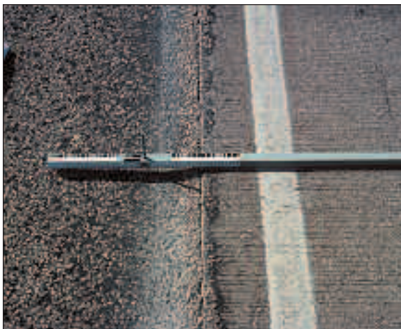
Figure 80: Distress Type JCP 13 Lane-To-Shoulder Dropoff
