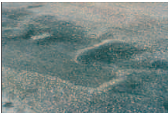
Figure 35: Distress Type ACP 10 Shoving in Pavement Surface
