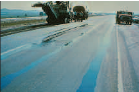
Figure 33: Distress Type ACP 9 Standing Water in Ruts
