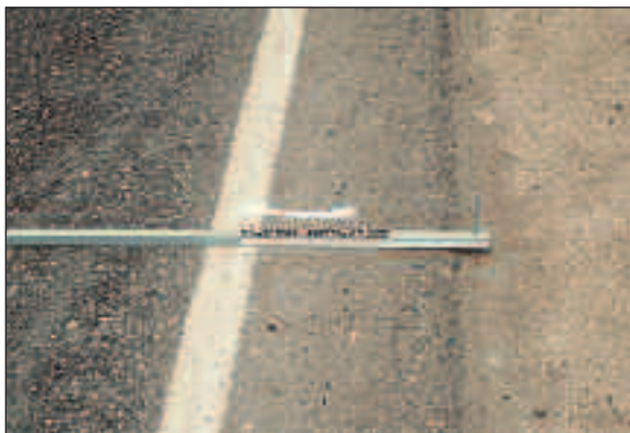
Figure 44: Distress Type ACP 14 Lane-to-Shoulder Dropoff
