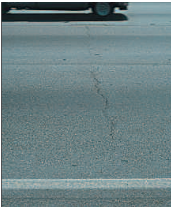
Figure 19: Distress Type ACP 6 Low Severity Transverse Cracking
