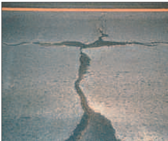
Figure 45: Distress Type ACP 15 Water Bleeding and Pumping
