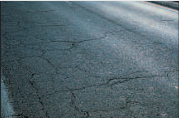
Figure 10: Distress Type ACP 2 High Severity Block Cracking
