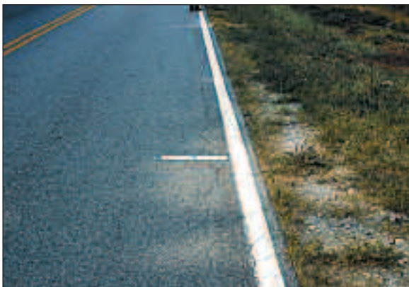
Figure 12: Distress Type ACP 3 Low Severity Edge Cracking
