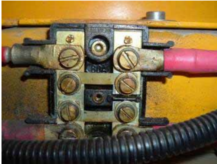
Figure 136. Trailer fuse block.
