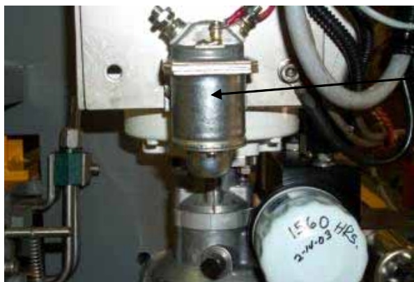
Figure 48. Solenoid mounted to hydraulic motor.
