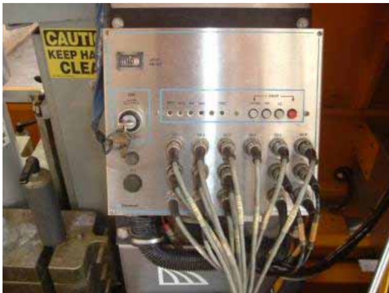
Figure 135. Power control box (board behind front panel).
