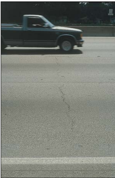
FIGURE 19 Distress Type ACP 6—Low Severity Transverse Cracking.
