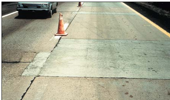
FIGURE 122 Distress Type CRCP 11—Low Severity PCC Patch.
