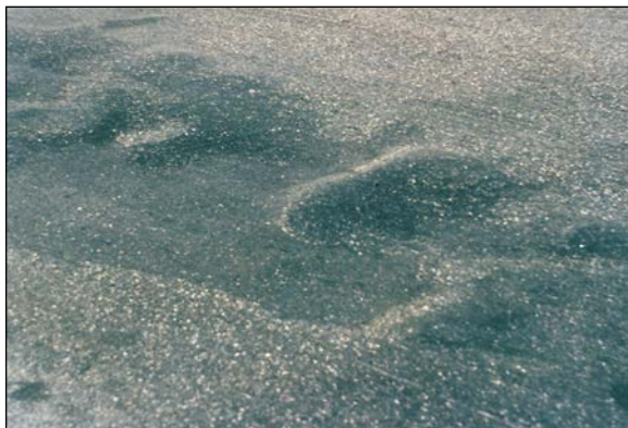
FIGURE 35 Distress Type ACP 10—Shoving in Pavement Surface.
