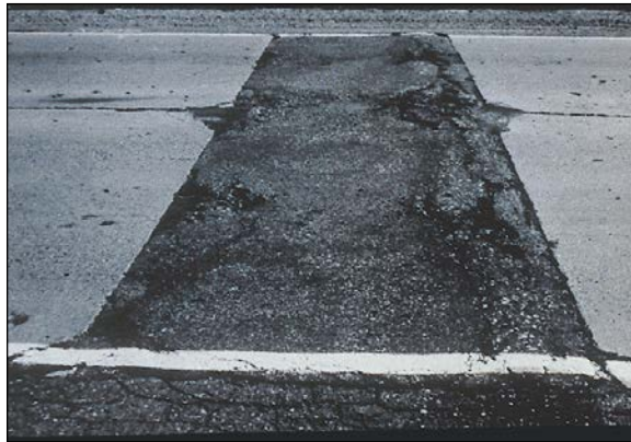
FIGURE 87 Distress Type JCP 15—Large, High Severity AC Patch.
