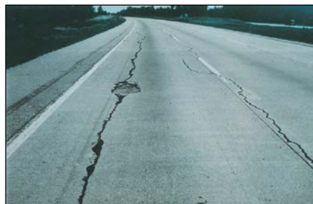
FIGURE 95 Distress Type CRCP 2—High Severity Longitudinal Cracking.
