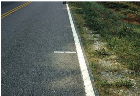
FIGURE 12 Distress Type ACP 3—Low Severity Edge Cracking.
