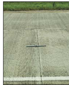
FIGURE 111 Distress Type CRCP 8—Low Severity Transverse Construction Joint Deterioration.
