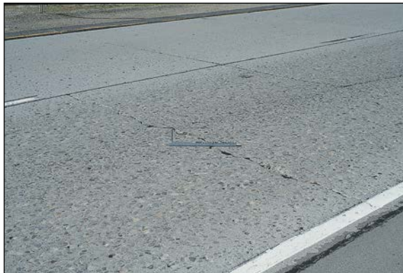
FIGURE 60 Distress Type JCP 4—High Severity Transverse Cracking.
