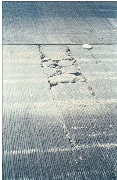
FIGURE 126 Distress Type CRCP 12—High Severity Punchouts.
