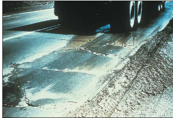
FIGURE 89 Distress Type JCP 16—Water Bleeding and Pumping.
