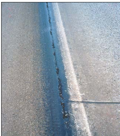
FIGURE 82 Distress Type JCP 14—Poorly Sealed Lane-to-Shoulder Separation.
