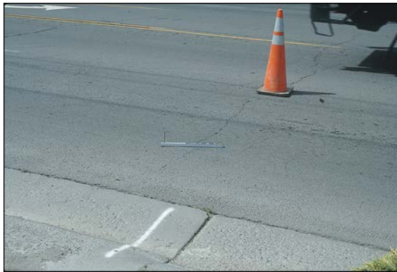
FIGURE 20 Distress Type ACP 6—Moderate Severity Transverse Cracking.
