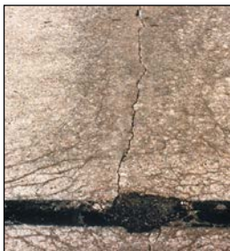
FIGURE 91 Distress Type CRCP 1— Moderate Severity “D” Cracking at Transverse Crack.
