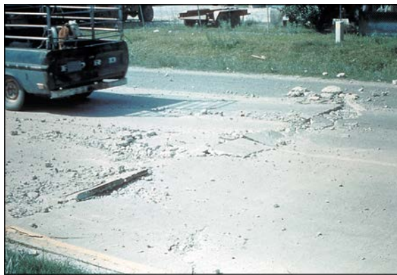
FIGURE 76 Distress Type JCP 11—A Blowup.
