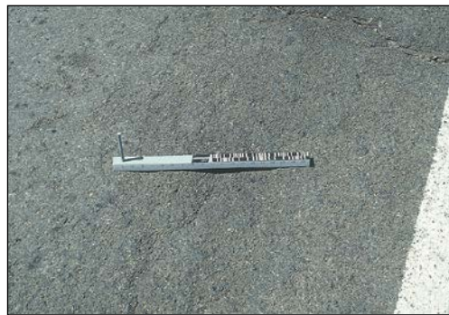
FIGURE 40 Distress Type ACP 13—Loss of Fine Aggregate.
