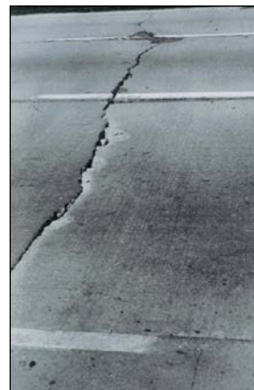
FIGURE 78 Distress Type JCP 12— Faulting of Transverse Cracks.
