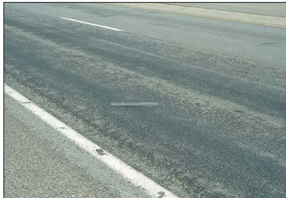
FIGURE 37 Distress Type ACP 11—Loss of Texture.
