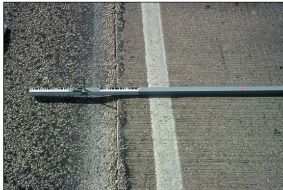
FIGURE 80 Distress Type JCP 13— Lane-to-Shoulder Dropoff.
