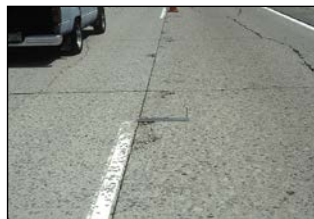
FIGURE 65 Distress Type JCP 6—High Severity Spalling of Longitudinal Joint.
