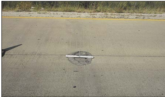
FIGURE 121 Distress Type CRCP 11—Moderate Severity AC Patch.
