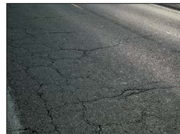
FIGURE 10 Distress Type ACP 2—High Severity Block Cracking.
