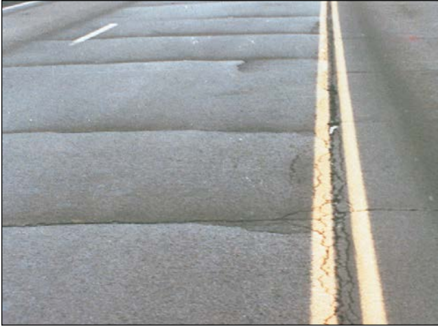
FIGURE 17 Distress Type ACP 5—High Severity Reflection Cracking at Joints.
