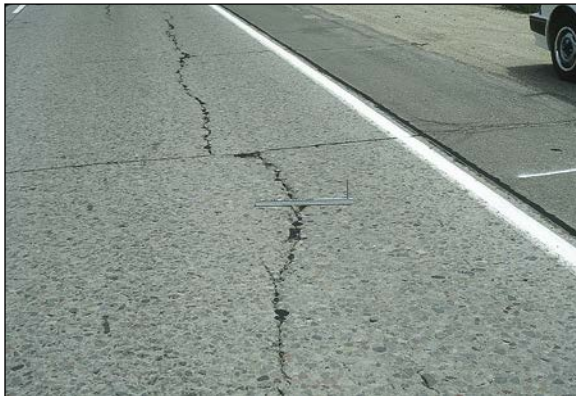
FIGURE 57 Distress Type JCP 3—High Severity Longitudinal Cracking.
