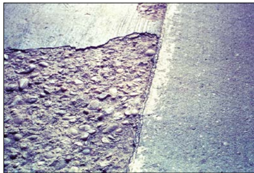
FIGURE 70 Distress Type JCP 8b—Scaling.
