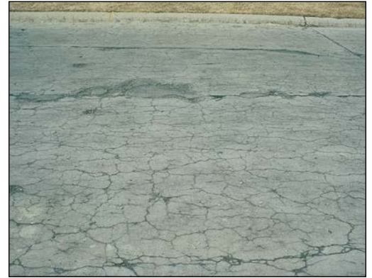
FIGURE 69 Distress Type JCP 8a—Map Cracking.
