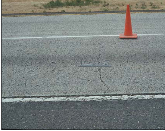
FIGURE 98 Distress Type CRCP 3—Low Severity Transverse Cracking.
