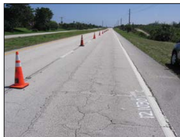
FIGURE 9 Distress Type ACP 2—Block Cracking with Fatigue Cracking in the Wheel Paths.
