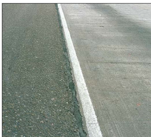
FIGURE 83 Distress Type JCP 14—Well-Sealed Lane-to-Shoulder Separation.
