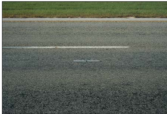
FIGURE 36 Distress Type ACP 11—Discoloration.
