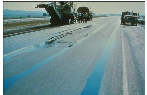
FIGURE 33 Distress Type ACP 9—Standing Water in Ruts.
