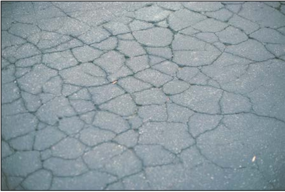
FIGURE 4 Distress Type ACP 1—Chicken Wire/ Alligator Pattern Cracking Typical in Fatigue Cracking.
