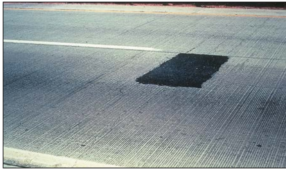
FIGURE 120 Distress Type CRCP 11—Low Severity AC Patch.
