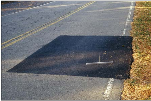
FIGURE 24 Distress Type ACP 7—Low Severity Patch.
