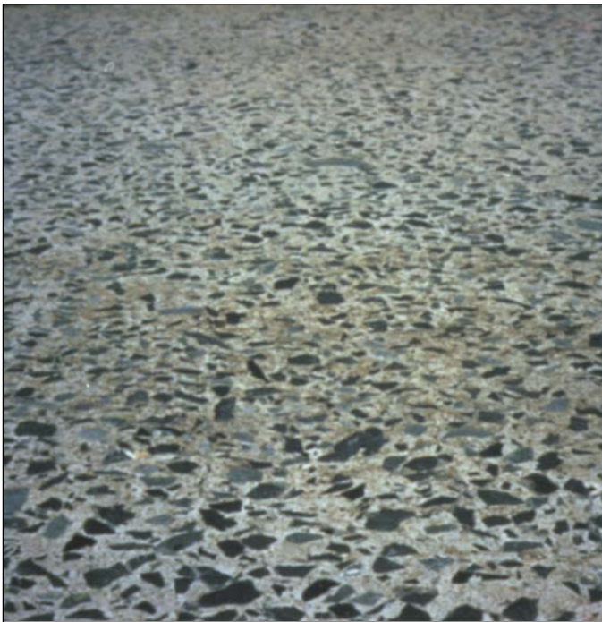
FIGURE 103 Distress Type CRCP 5—Polished Aggregate.
