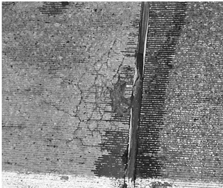
Figure 7. Map cracking observed in FS section in 1997.
